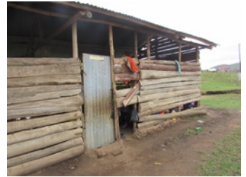
The existing school block to be replaced by the new 5 classroom block.
